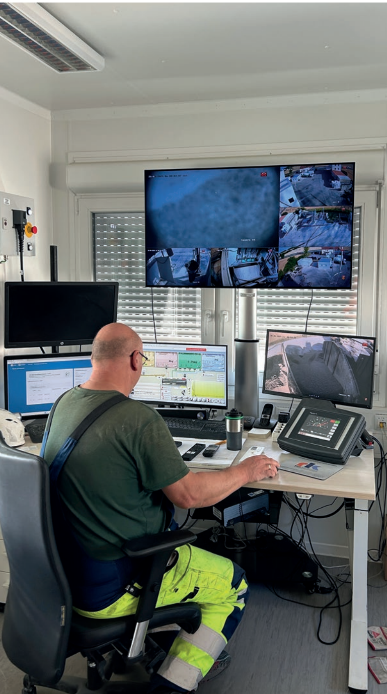
The mixing master building and the entire plant control system were completely modernised in the course of the conversion.
