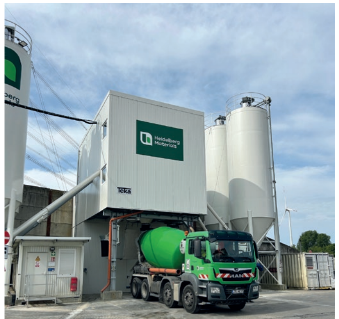
A new Teka Mixomat THZ 3000 mixing plant was put into operation at the Lindenberg plant in Ahrensfelde.
