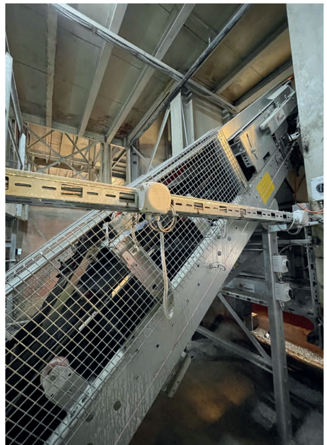
The weigh belts load a cross conveyor arranged underneath, which is designed as a VHV cover belt. The carrying belt pulls off horizontally at the feed point and then rises to a slope of 41° using the patented VHV flexi drum.
