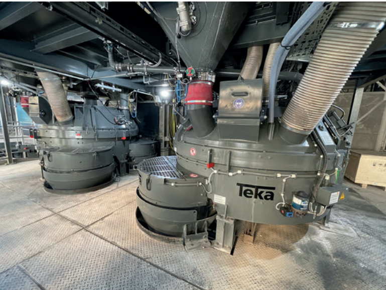
The two THT G-2-V turbine mixers from Teka are the centre-piece of the new concrete mixing plant.
