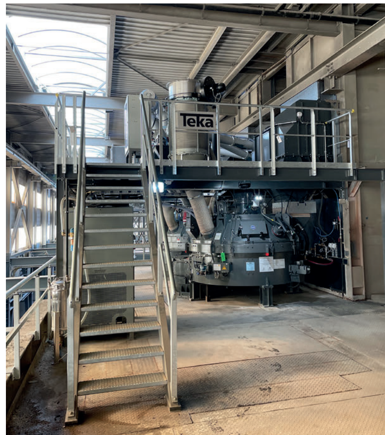
View of the new mixing plant at Lithonplus
