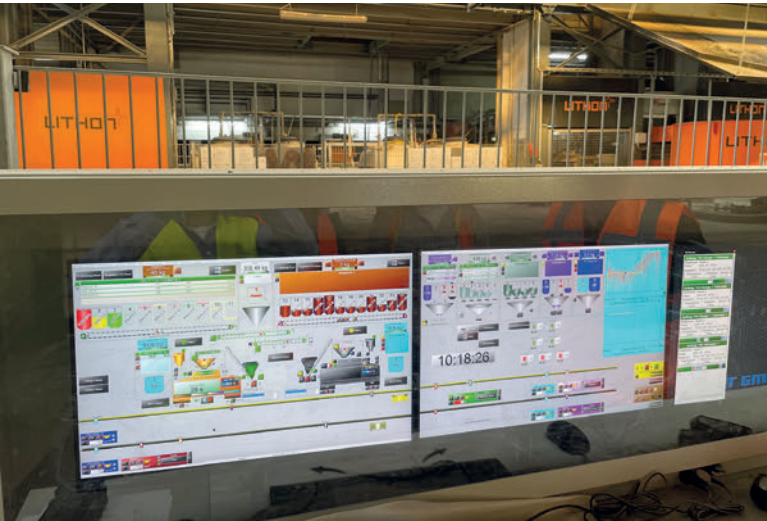
The complete concrete mixing plant is displayed via a visualisation level.
