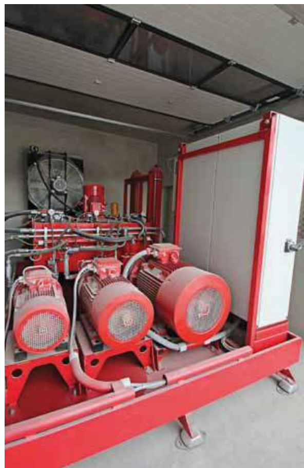
The complete hydraulic system had to be installed in a separate service room beside the actual production line
