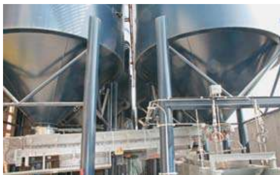
Fig. 3 The aggregates are transported from the new silos to the concrete mixing tower by weigh belts.
